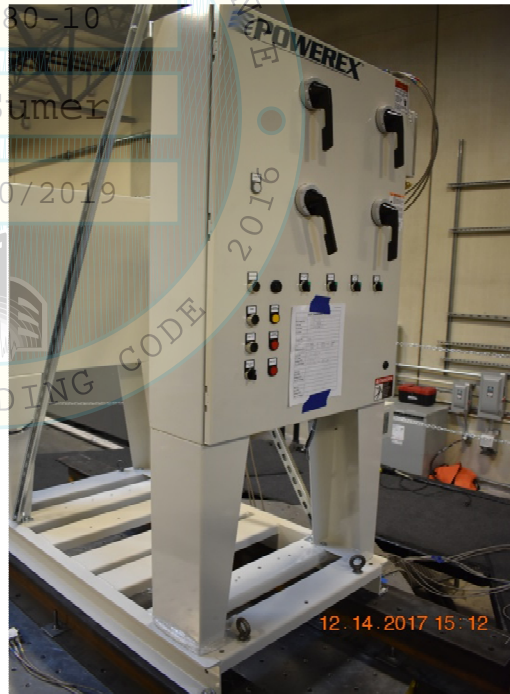
UUT14b - quadruplex panel
