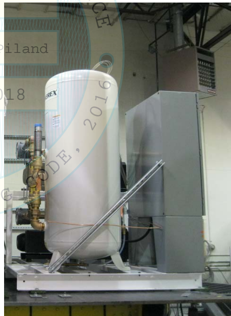
UUT3, view from left
