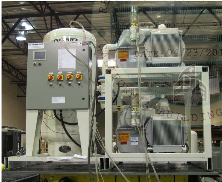
UUT2, view from front
