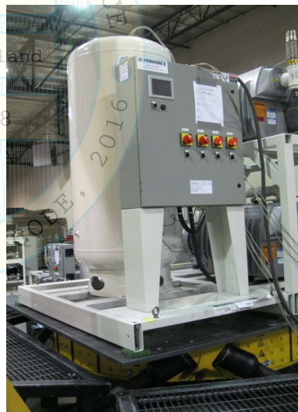
UUT2, view from left
