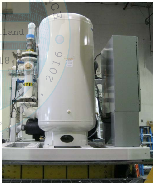
UUT4, view from left
